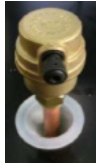
AERATOR - LOCATED ON TOP OF BOILER
