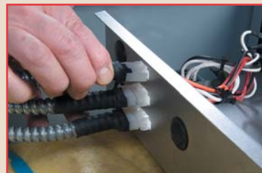
Controls come standard with factory wiring and plug 'n play harnesses
